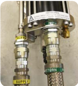
Coldhead flex hose connections
